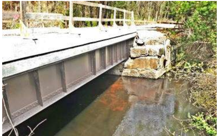
Phase 2A Bridge being restored. Original riveted steel beams with native cut granite piers and new concrete top shade Nashoba Brook (see Phase 2A, next page).
