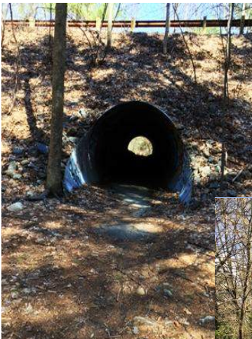
The contractor expects to replace this old culvert under Powder Mill Road with a new, larger, culvert this summer.
