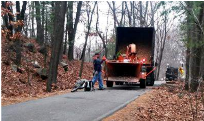
Chelmsford DPW removing debris and small dead trees. BPAC appreciates the multi-day efforts of the DPW staff to maintain the trail in Chelmsford.
