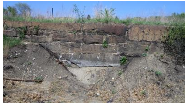
A portion of the wall further down the track was recently excavated revealing the entire wall down to its foundation.
